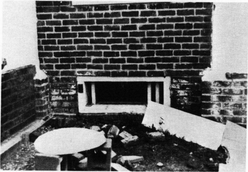
Figure III-69. Ventilation of Fairfax crawl space.
